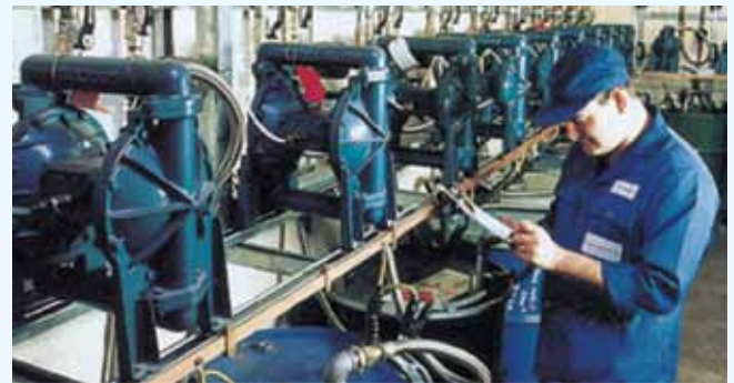
Fully automated Rexson ink manufacturing plant. Blagdon 25 metallic pumps are used for mixing and recirculation.
