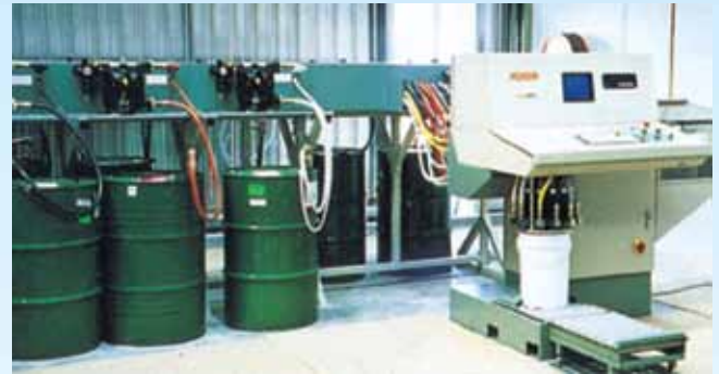
An ink pumping and mixing plant at Amcor Packaging in Australia using Blagdon 15 moulded pumps.
