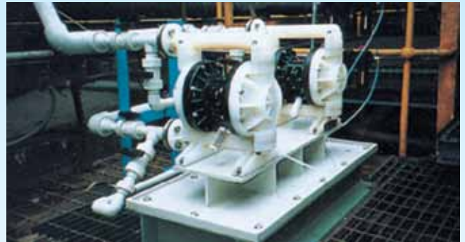
Blagdon 25 moulded Kynar pumps transferring hydrofluoric acid.
