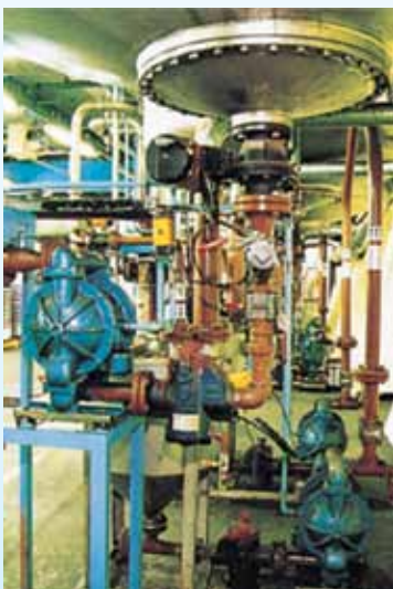
Part of the filtration process at a major multi-national paint manufacturer where Blagdon 50 pumps are used to supply the fully automated filling line.
