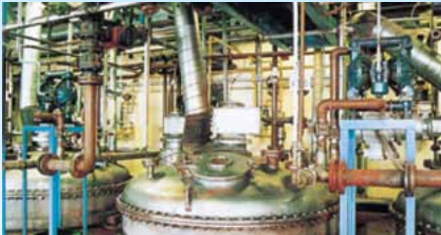
Blagdon 50 pumps feeding a ring main for final blending at a coatings producer.
