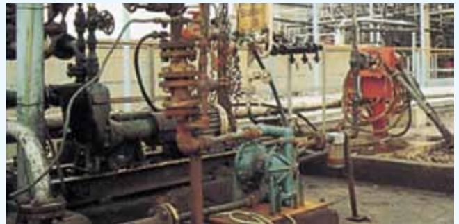
Blagdon 25 metallic pump at a major chemical plant in Northern England.
