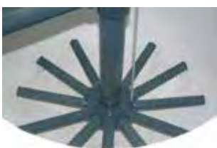
Collector arms detail
