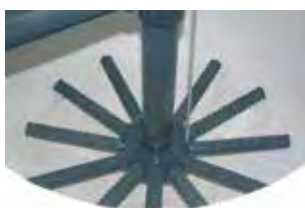
Collector arms detail
